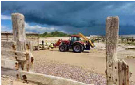
Environment Agency operatives, seen through a gap in a groyne, dismantle a dilapidated section of breakwater.
