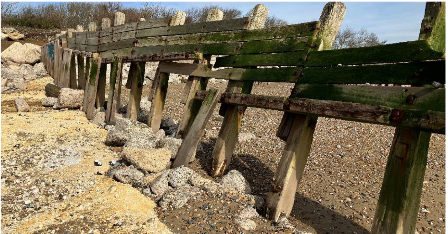
Timber groyne at Climping beach no longer retaining shingle and posing a hazard
